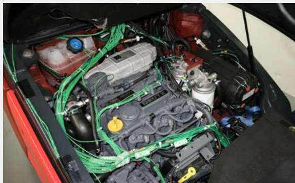
Fig. 7: The temperature and pressure sensors are installed in the specified locations in the engine compartment. The green cabling shows routing of the Type K thermocouple sensors to the measurement modules located outside the confined engine compartment.
